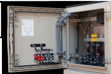
Industrial power supply and metering panel, housed in a plastic box
