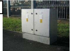
Stainless steel traffic equipment cabinet
