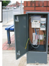
Power supply and metering for traffic signal equipment
